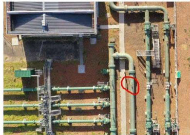
Figure 3. OverView of site and location of LineVu installation
